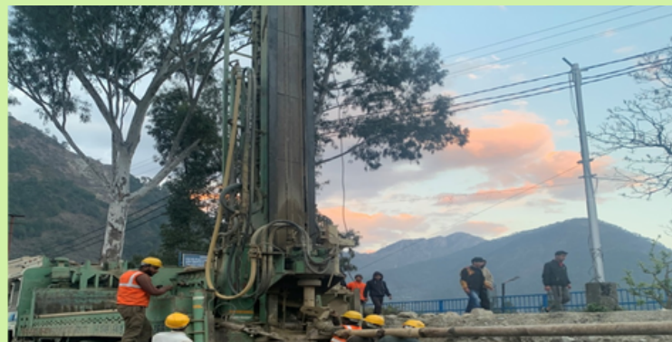
Arrangement of Drilling Rig which was used for drilling of curtain grout holes is seen in operation.
