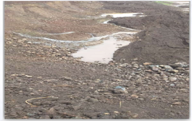
Fig.1- Downstream Slope Failure
