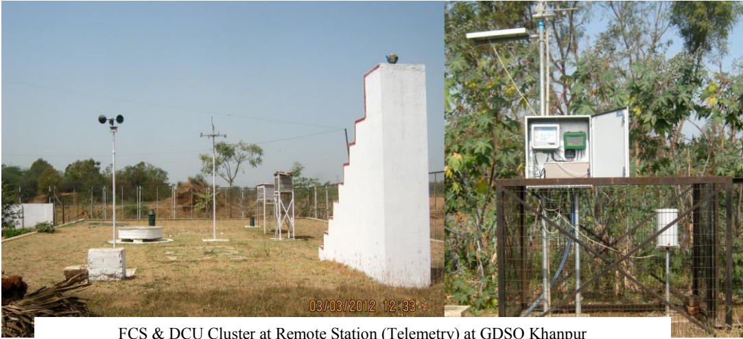
FCS & DCU Cluster at Remote Station (Telemetry) at GDSQ Khanpur
