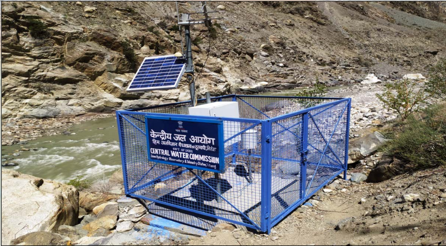
TITANG B-TYPE TELEMETRY STATION, SHD, CWC, SHIMLA ON RIVER SATLUJ
