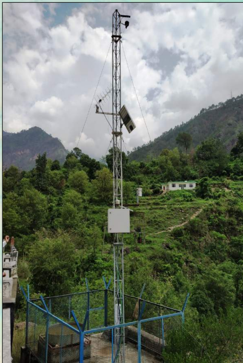
PANDOWA D-TYPE TELEMETRY STATION, SHD, CWC ON RIVER SATLUJ
